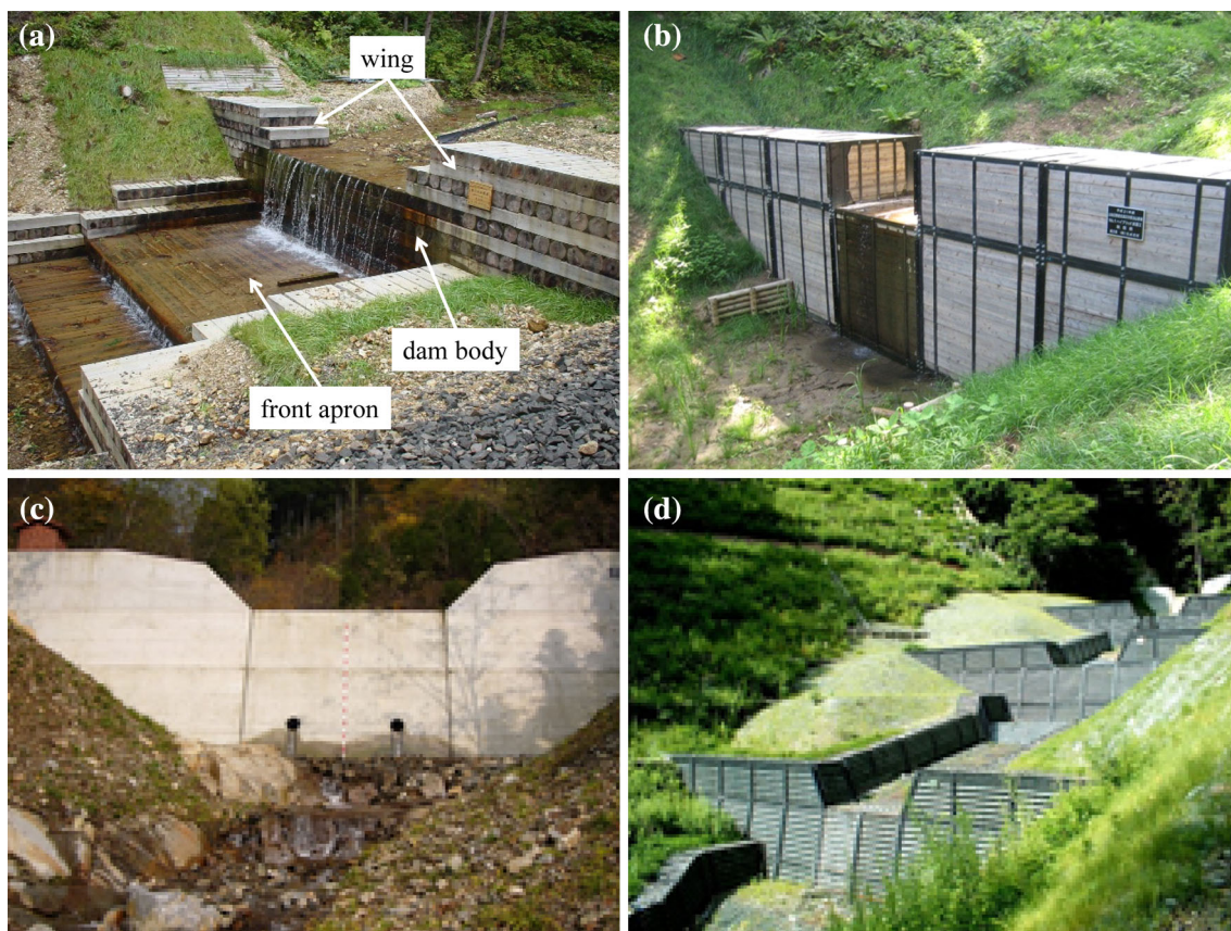
Fig. 1 Types of check dam a All-wood timber check dam, b hybrid timber check dam, c Concrete check dam, d Steel check dam
