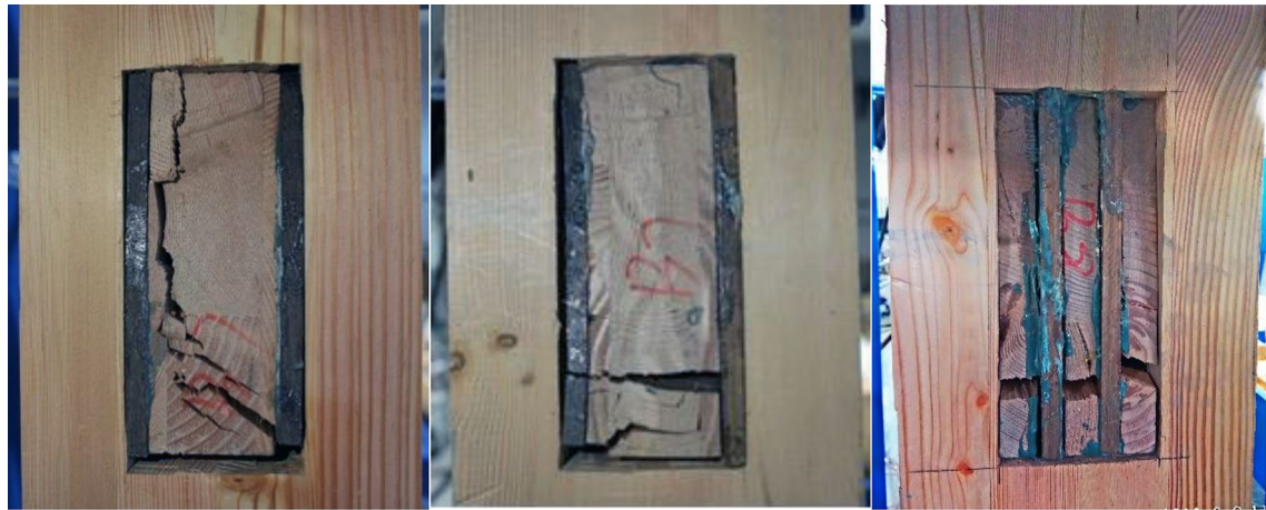
Fig. 6 Cracks observed in the reinforced mortise and tenon joints
